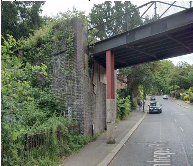
Figure 2: View looking south along Stanhope Road showing temporary structural props on east footway.
